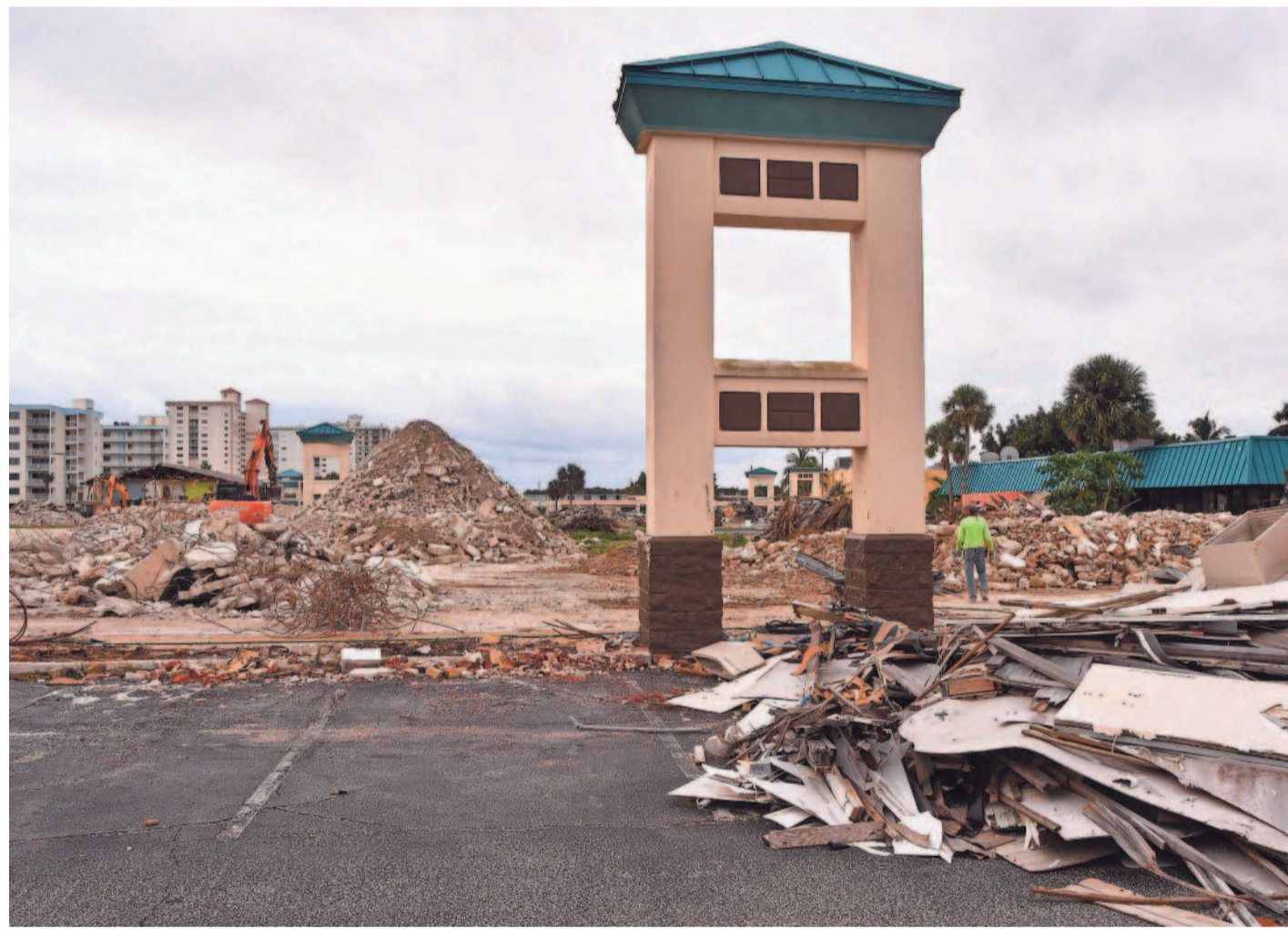
The demolition of the International Palms in Cocoa Beach has begun. Replacing it will be a $300M Westin luxury resort at the site. Driftwood Capital bought International Palms for $23 million in October 2016. MALCOLM DENEMARK/FLORIDA TODAY
